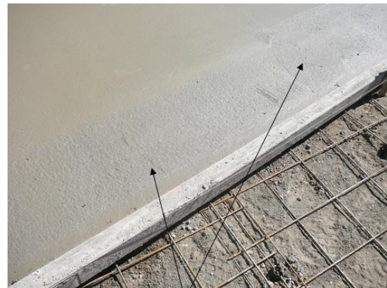
Plastic Shrinkage cracking
