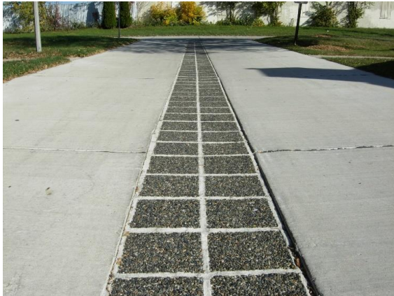
Figure 24.2 – Porous Concrete Pavement in the Middle Strip of Two Parallel Concrete Pavements 24.2
